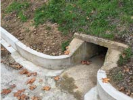
Channelling barriers for amphibians in hydraulic crossings under the roads
